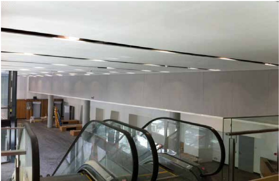
| The Supercoil long span smoke curtain installed at the Brisbane Convention & Entertainment Centre
